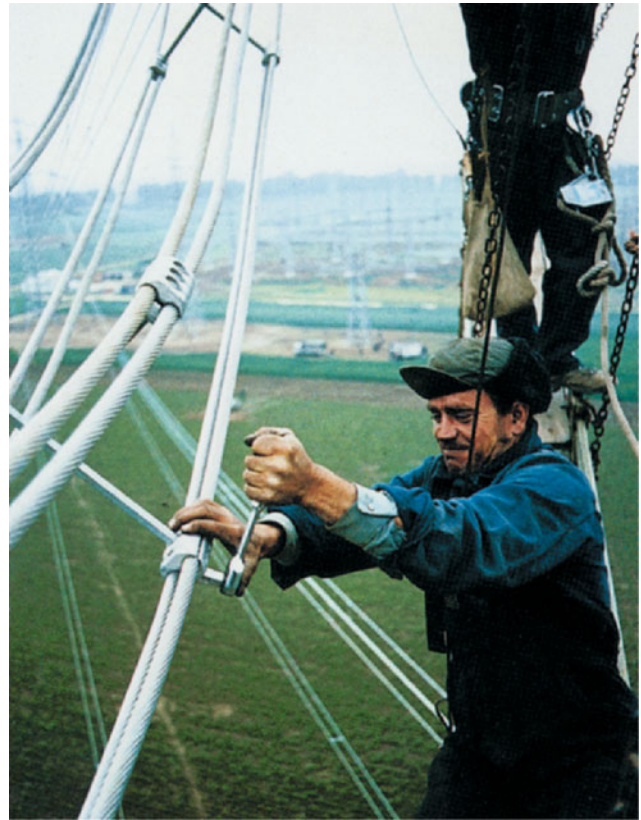
Fig. 5.37 Installation of a high voltage power line. In this picture each phase of the three phase current is transmitted by 4 cables arranged in quadratic form, connected by the diagonal bracket seen in the upper part of the picture. Each cable consists of two wires. The technician just fixes the connection between these wires (with kind permission by information center of the Elektrizitätswirtschaft Frankfurt)
